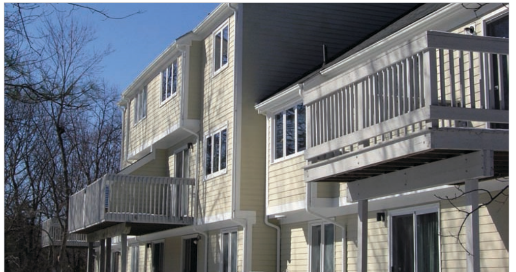
SPS replaced Drummer Boy Home’s original wooden clapboard and trim with moisture- and insect-resistant fiber-cement clapboard and trim. SPS specializes in managing the kind of large-scale building envelope work that many associations are now facing.
